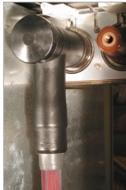
CB innstalled in Siemens switch type 8DJ-10.
